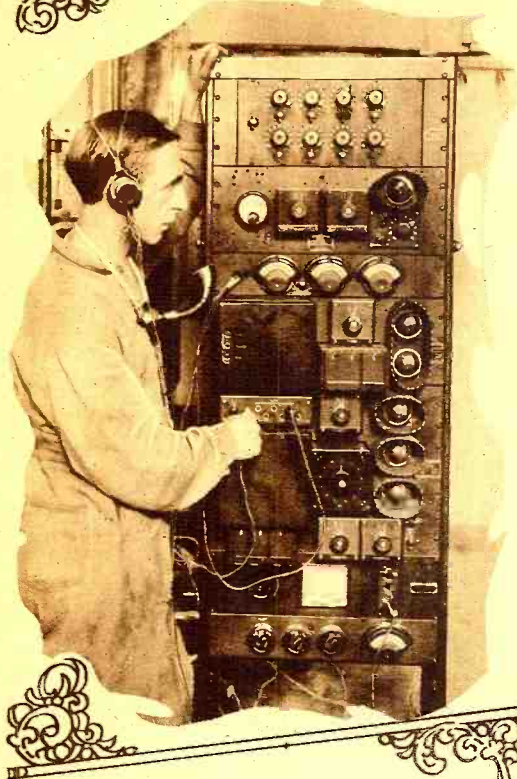
Above is shown the control board for the hotel public address system. Through the agency of this system it is possible to introduce any program being given in the studio of WRNY into any of the public rooms of the hotel or to pick up speech from any room in the hotel and put it on the air through WRNY.
